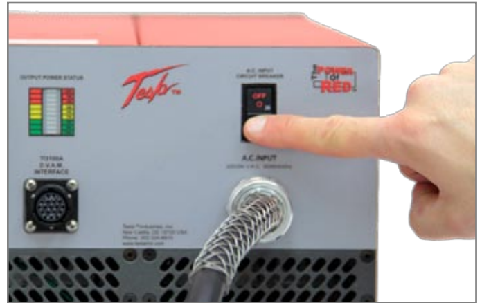
Figure 3.9.1 - Turning On AC Input Circuit Breaker
