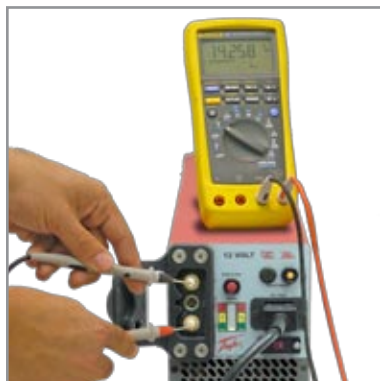
Figure 3.8.2 – Testing DC Receptacle
